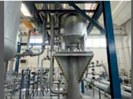
The tanks with electronic scales and emptying valves.
